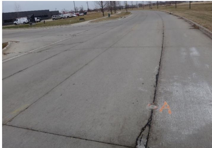
Figure 80. Field view of distressed joint
