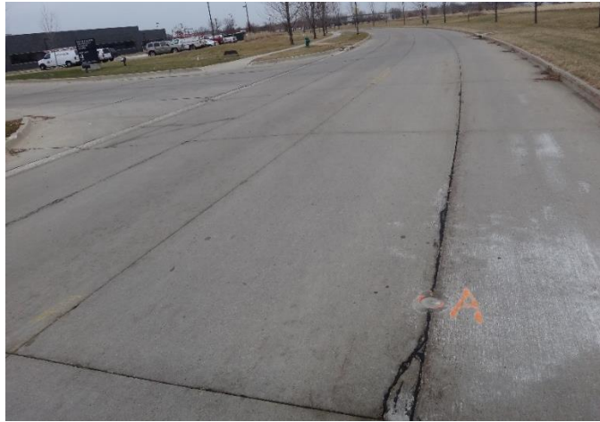
Figure 57. Field view of core 4 location showing joint distress
