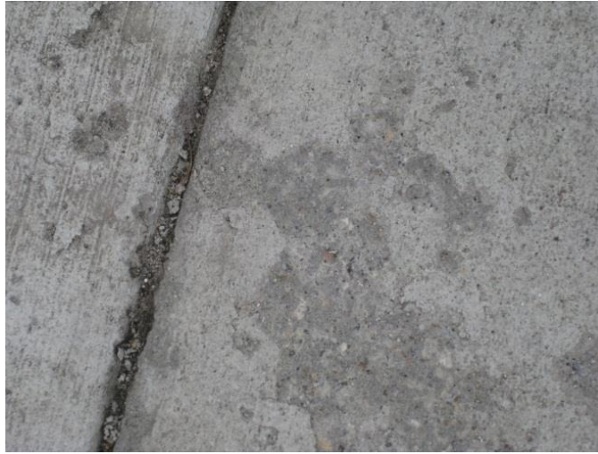
Figure 10. Salt scaled concrete sidewalk
