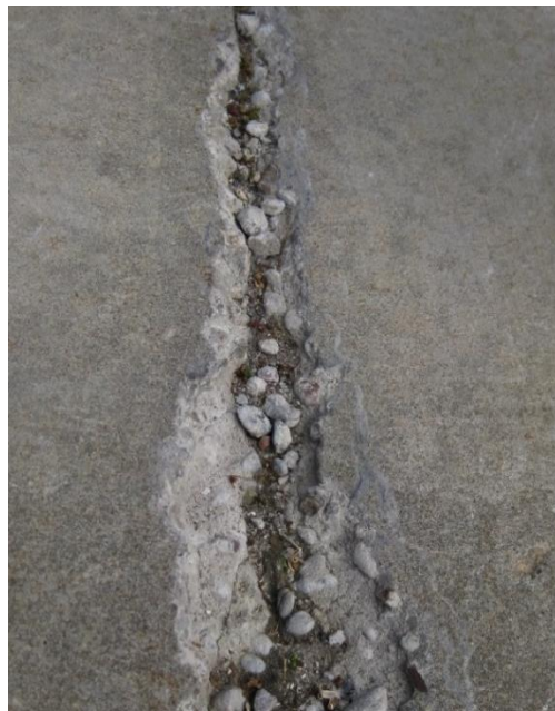
Figure 41. Field observation of joint deterioration
