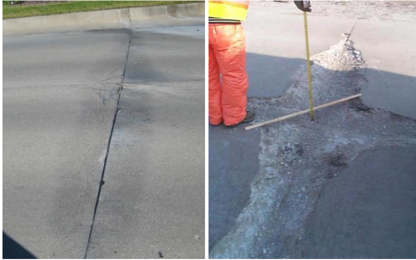
Figure 69. Deteriorated joint in concrete pavement
